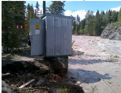
Elbow River at Bragg Creek 2013
